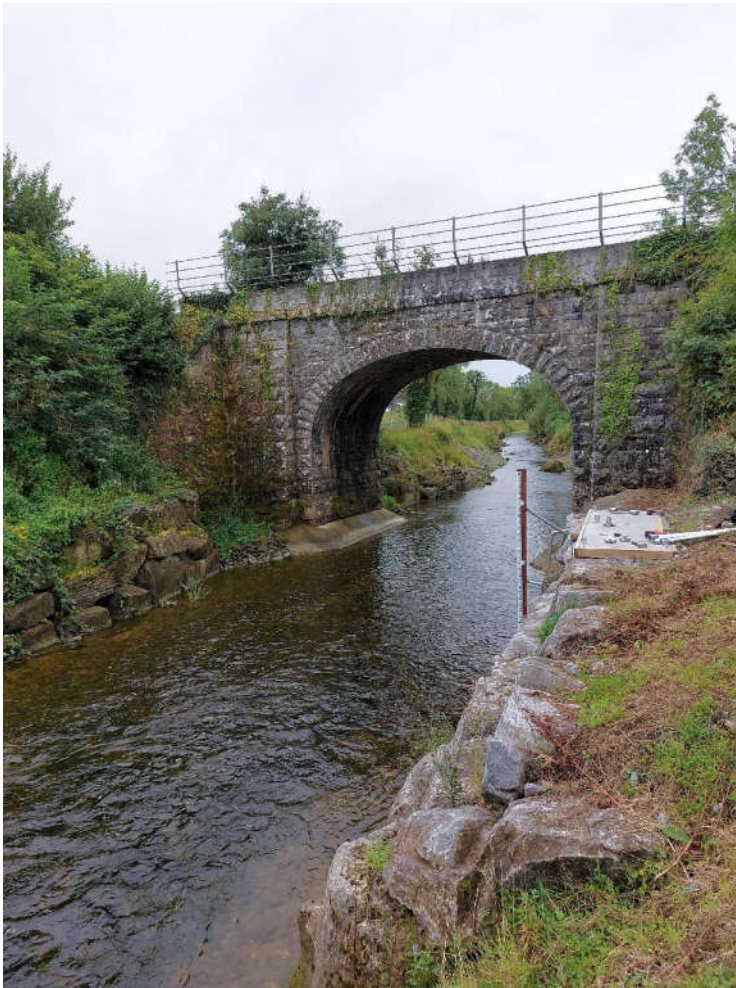
Plate 1 OPW Hydrometric Station Craughwell 29007 (facing west)
